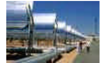
Solar Power Generating Plants
