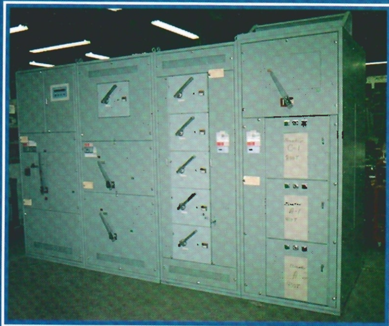
Indoor switchboard with bolted pressure, vacubreak and draw out switches
