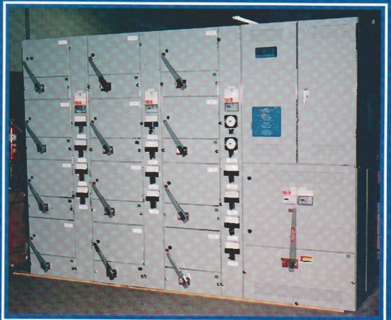
NEMA 1, 120/240, 4000 Amp, 1 phase 3 wire metering with main switch and bolted pressure switches
